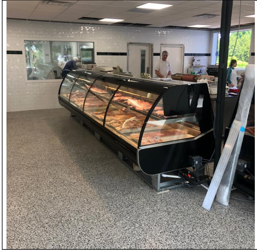
Figure 7 – Post Project Arneg Refrigeration Case
