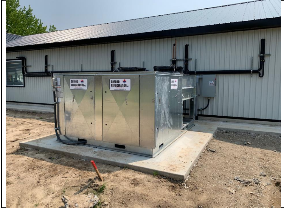
Figure 9 – Post-Project Condensers Oxford Refrigeration System
