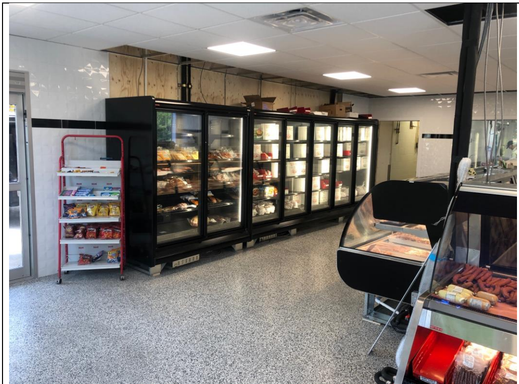
Figure 8 – Post Project Arneg refrigeration case installation
